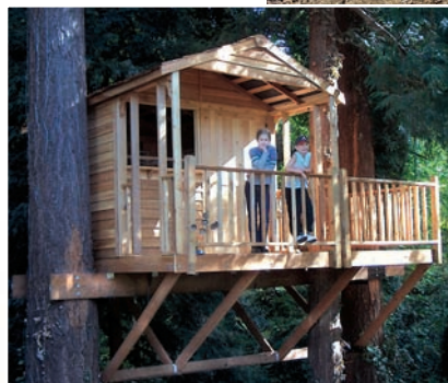
A strong support system was planned to ensure that this grown-up "treehouse" is not only fun for all, but sturdy enough to be safe. 8' x 12' clubhouse, built by the Kellog family of Vancouver, Washington
